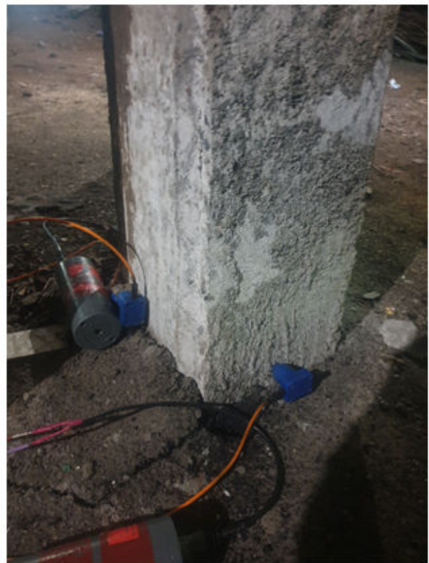
Figure 4: Example of installation of horizontal and vertical geophones gs20dx and single-channel digital recorders Texan (RefTek-125A) on piles.
