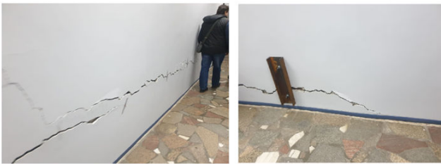
Figure 3: Shows cracks on the 1 st floor.
