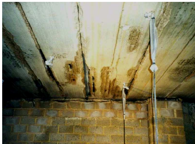
Figure 2. Cavities at the centre of the planks cause discontinuity of the thermal transfer during fire condition
