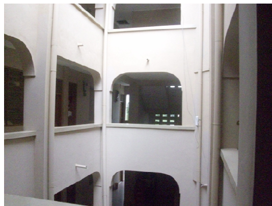
Fig 4 A view showing the inefficient courtyard of the hostel
